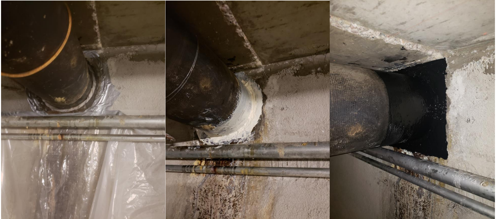
Above is the 2 nd pipe sleeve with the poly fabric and EP-990 applied, then the 2K Epoxy Sealant, then on the end it the Urethane Coating we added.
